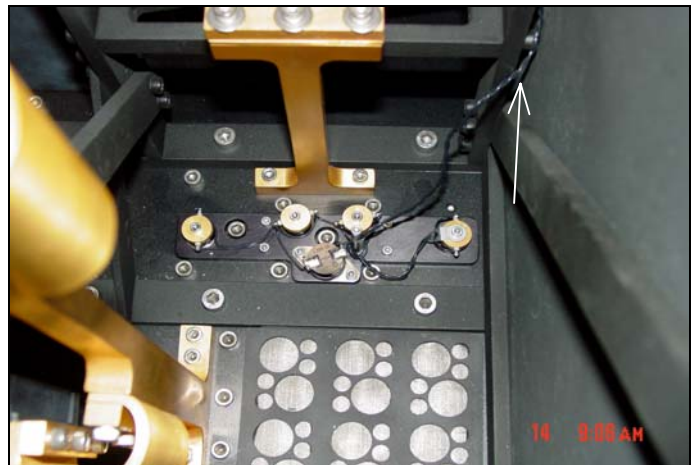
24. Mating Dewar - CWS heater circuit, 1 heater button can be relocated to the getter box. The connector # J 11 is between the frame and shield, see arrow.
